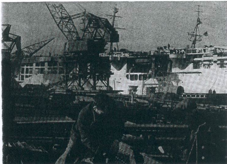
Work in progress on the conversion of the RAPANA as a M.A.C.
